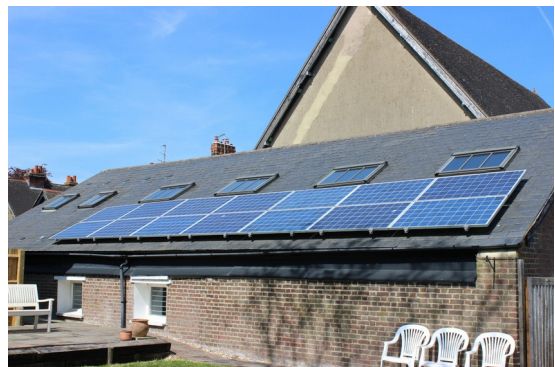
Solar panels on the roof of High Street Baptist Church, Tring
